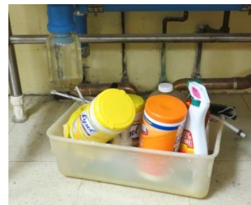
Figure 47: Chemicals on Floor in Secondary Containment
