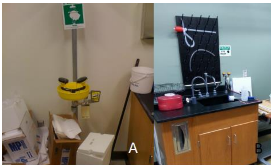
Figure 14: What qualifies as an obstructed safety shower or eyewash? A-Obviously obstructed combination unit. Storing items in front of a safety shower or eyewash is an obvious violation of lab safety procedures. B-Subtle obstruction of eyewash. Anything that can impede access to an eyewash or a safety shower is a violation of lab safety procedures. While picture B does not seem serious, a lab worker that cannot see due to having hazardous materials in their eyes could have trouble accessing the drench hose in this case. The red outline area on this sink may not have anything placed in it.
